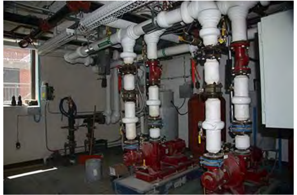
Ground source heat pump
