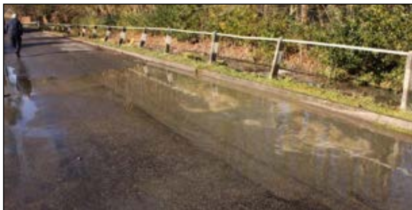
Figure 18: Sewer overflow in Berry Lane, January 2014
