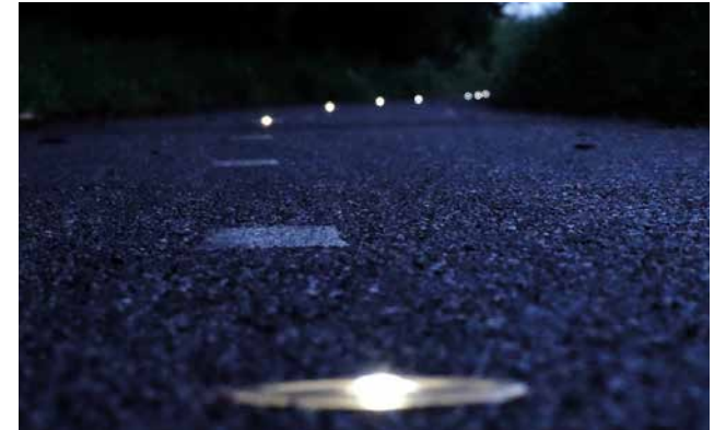
Figure 64: Example of a foot/cycle path which is lit by solar cat's-eye providing some light for pedestrian and cyclists without creating any disturbance to the nearby properties or unacceptable levels of light pollution.
