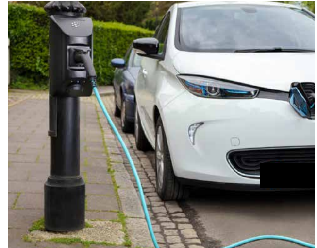
Figure 96: Example of on-street electric vehicle charging points.
