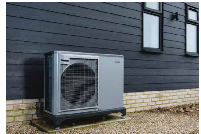
Figure 93: Example of an electric heat pump that is placed to the back of the house, whilst its grey colour blends well with the black weatherboarding of the property.
