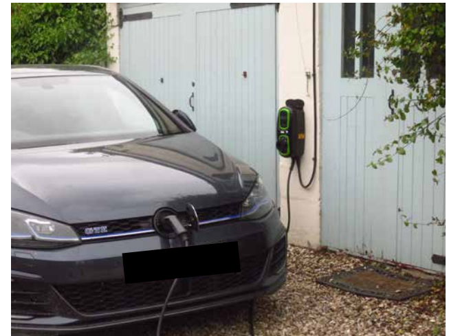
Figure 98: Local example of off-street electric vehicle charging point.
