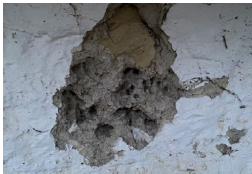
Fig 5. Section of cob wall in poor condition
